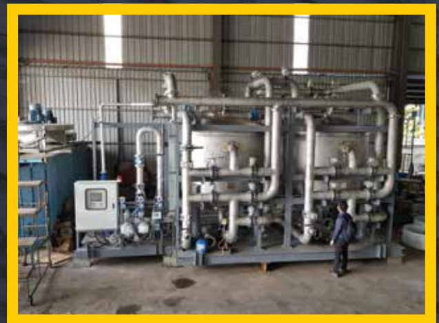
3,600 m 3 /day Sand Filtration
