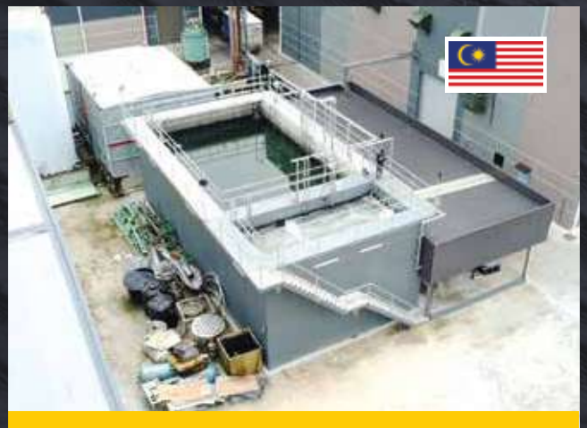
SBR Technology at Flavor Processing Plant
