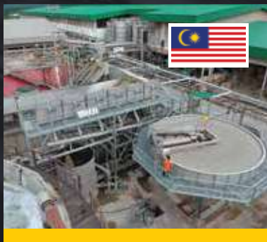
19,200 m 3 /d Paper Mill Processing WWTP
