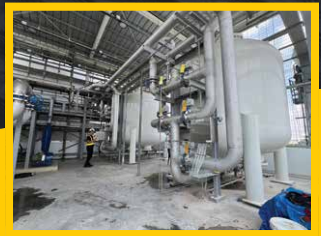
6,000 m 3 /day Process Water System
