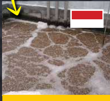
2,000 m 3 /d MBBR Technology (Oleochemical Plant)
